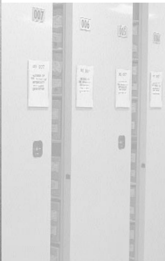
During a fire alarm and at night, the mobile system will leave 4- to 6-inch spaces between the carriages to serve as flues, which reduce the time it takes to put out a fire and the amount of fire damage.
