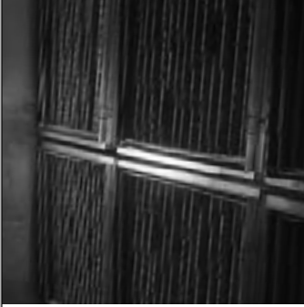
Pleated degas filters remove gaseous pollutants from the records storage areas.
