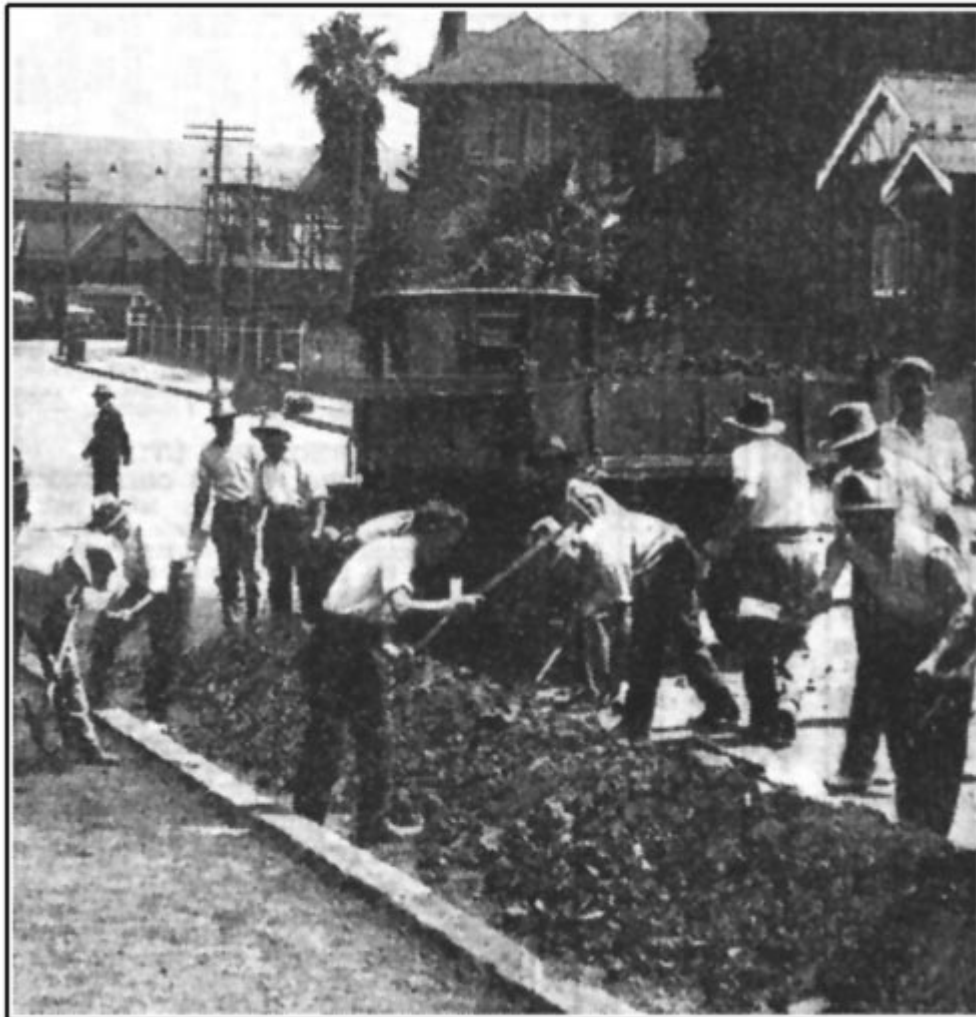
The construction of new footways is now well in hand in Hunter-street, Petersham.
